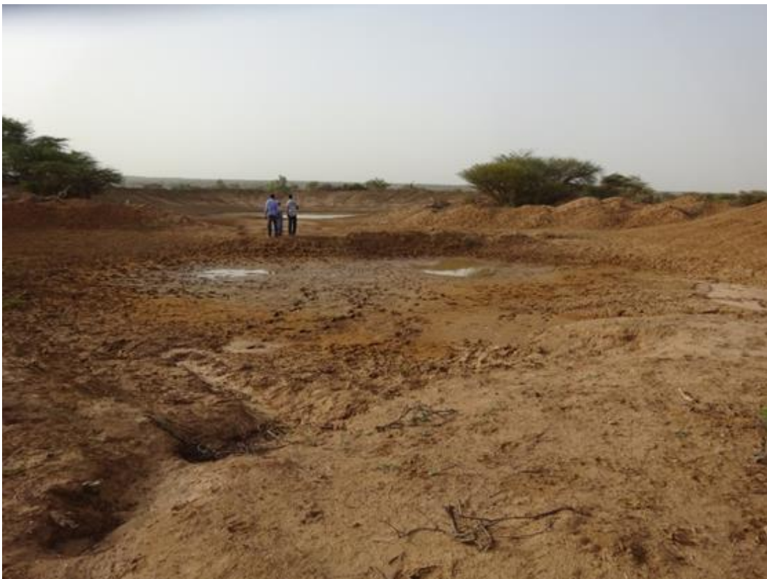
Photo The inlet of the rehabilitated 'bailey' earthen dam in Hareed village, Somaliland.
