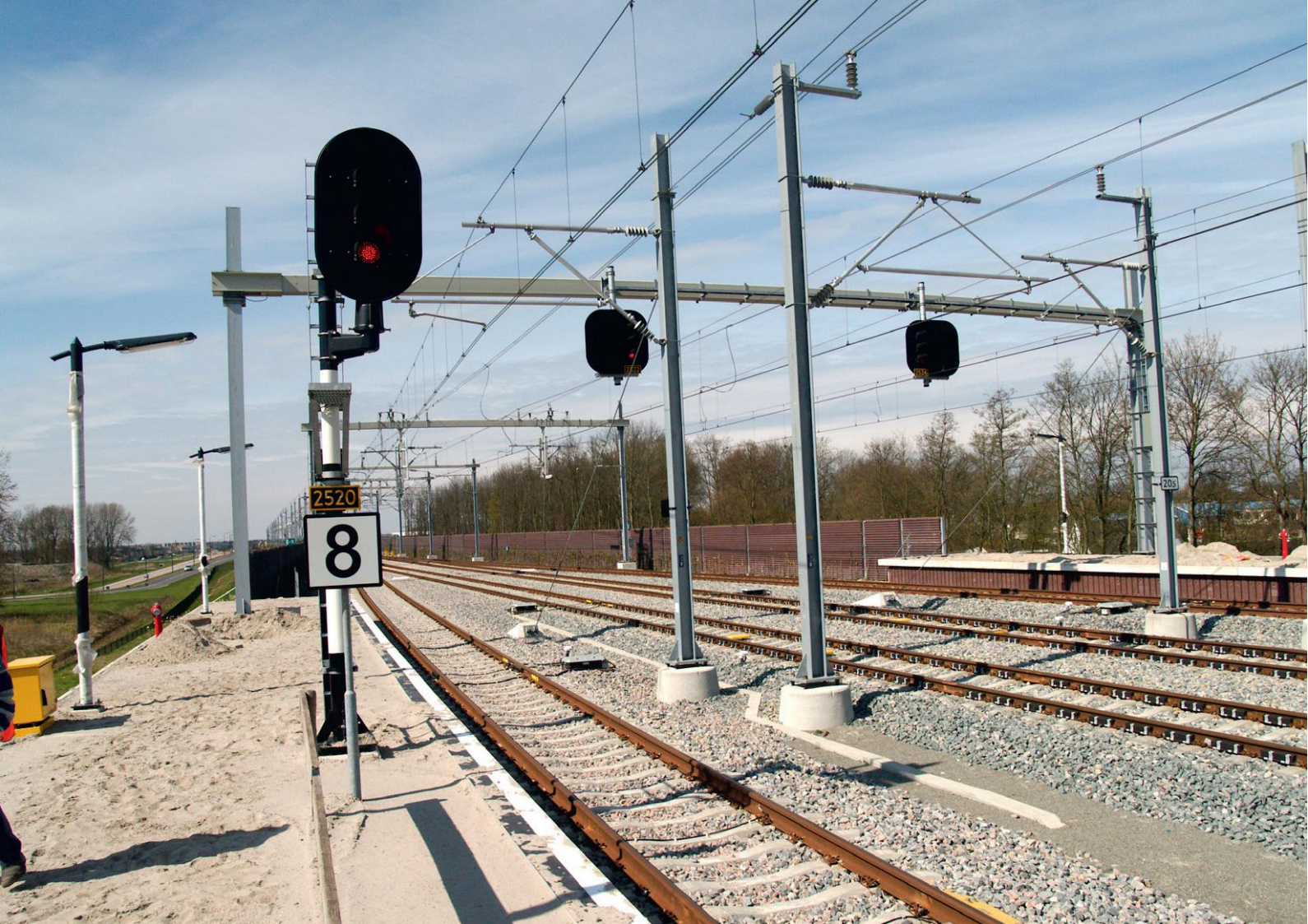
The Hanzelijn railway line is equipped with ERTMS and the current train protection system (dual signalling).
