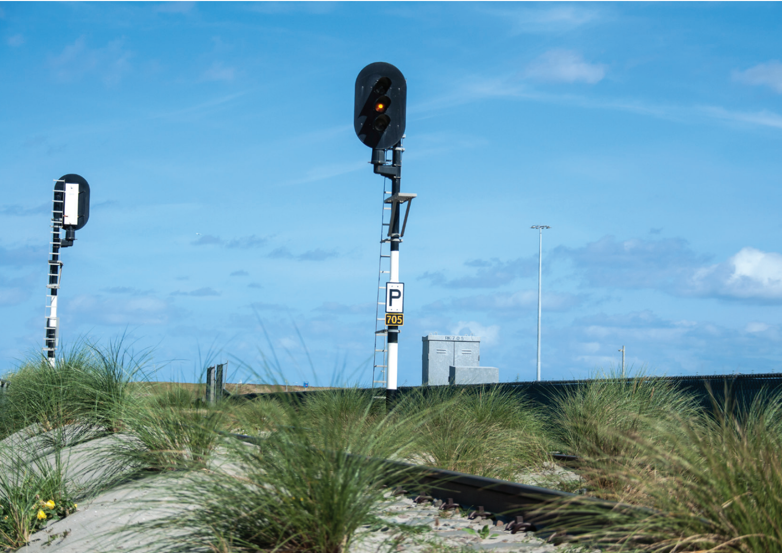
The Port Railway Line (Havenspoorlijn) is fitted with ERTMS Level 1
