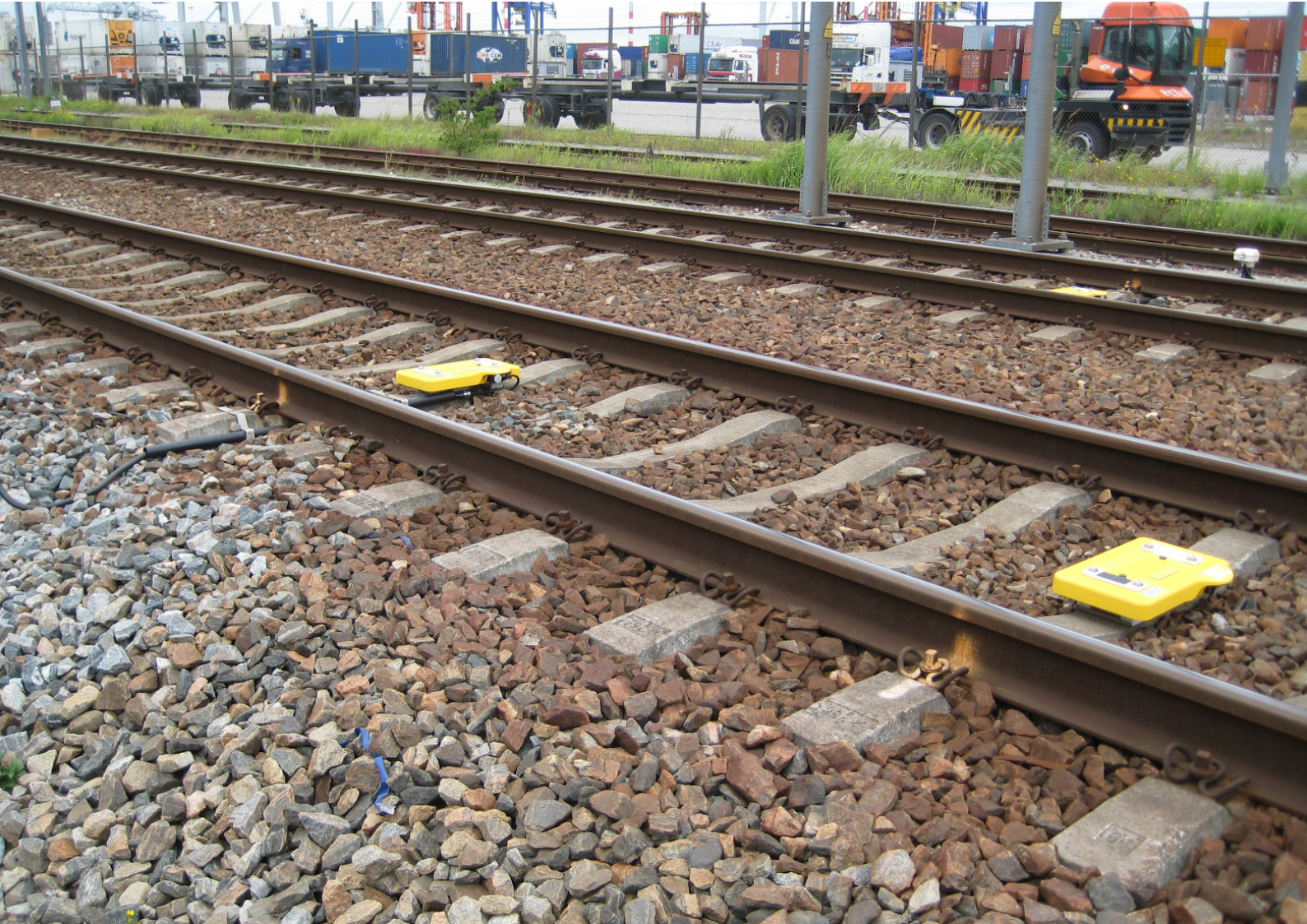
Eurobalises in the railway. These function as beacons within ERTMS.
