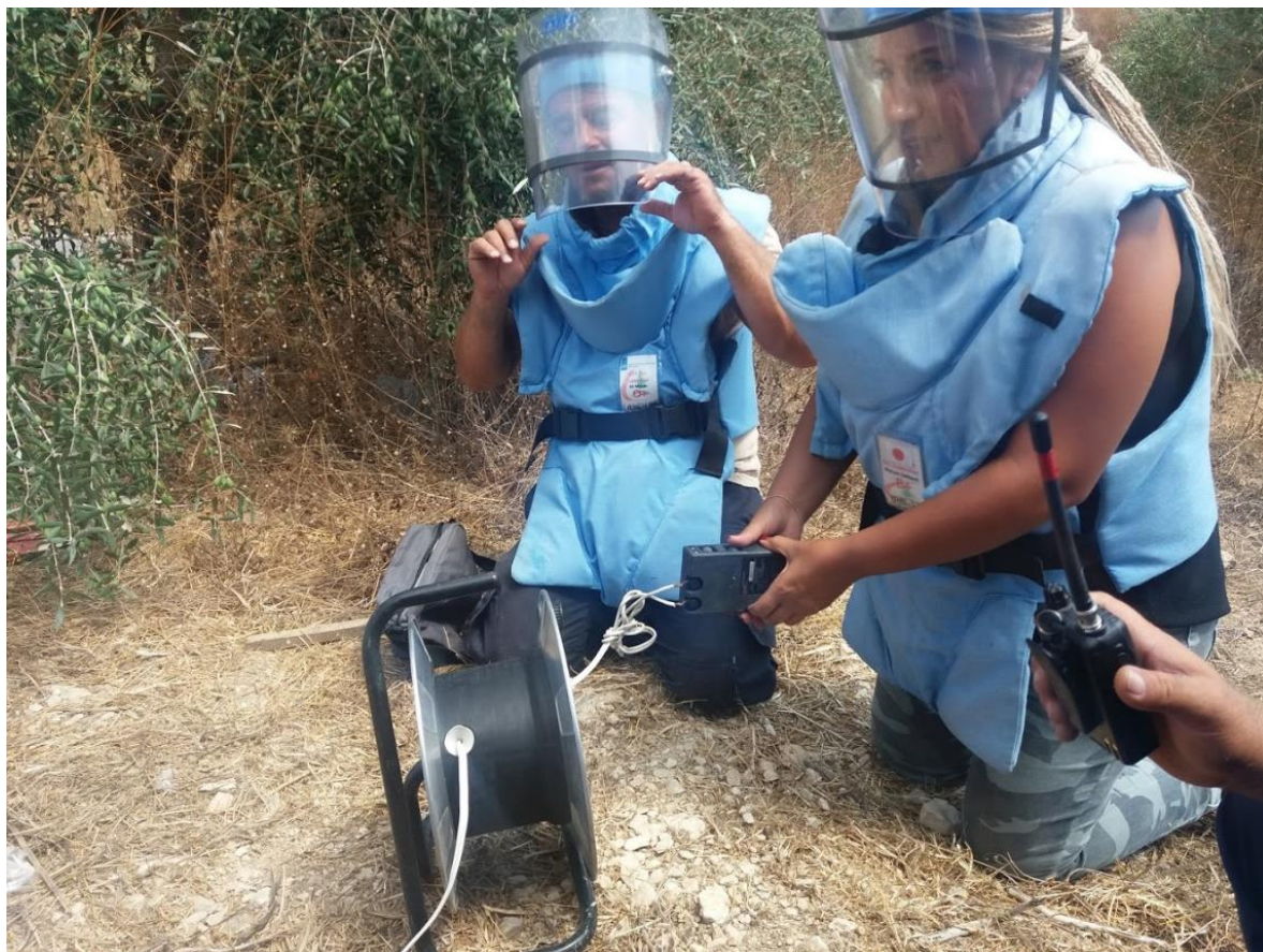
FIGURE 4. DEMOLITION OF CLUSTER MUNITION BY LAMINDA (SUPPORTED BY DCA), LEBANON (PHOTO: WELMOET WELS)
