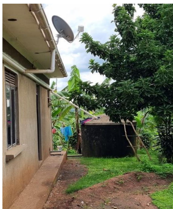
Rainwater harvesting system installed with project assistance
